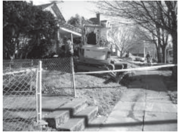
Digging up our sewer line and repairing the sidewalks on the same day
