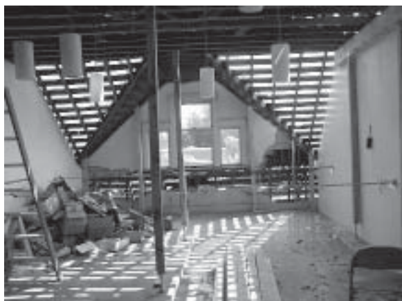
Pre-renovation pigeon mourage
