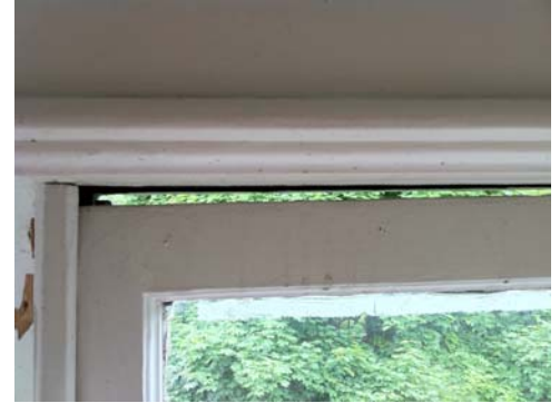
Eight windows had gaps like this. take note: this is in fully closed position
